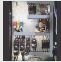
Electrical Cubicle Monitors Power Management
